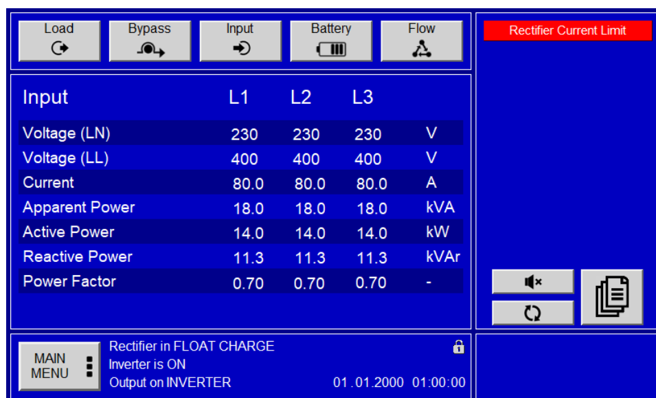
Figure 3-7 LEON-A Series UPS Touch Screen Panel - AC Input Measurements
