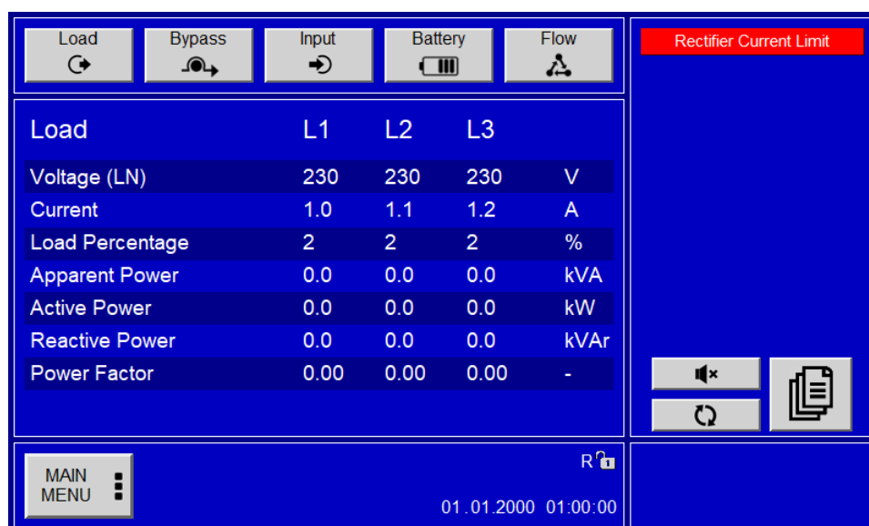
Figure 3-5 LEON-A Series UPS Touch Screen Panel - Load Measurements
