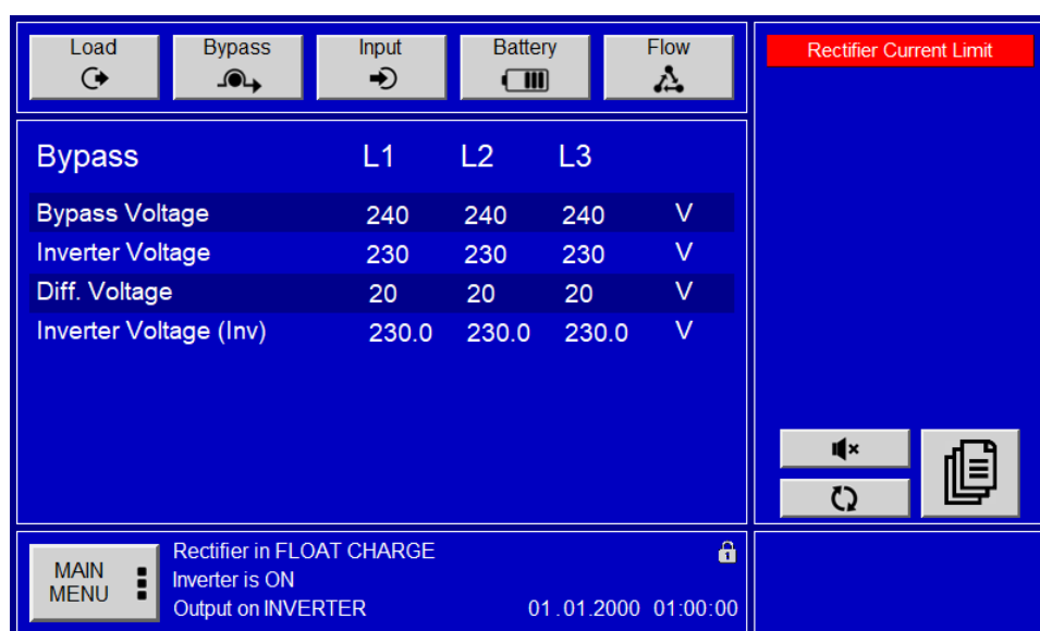
Figure 3-6 LEON-A Series UPS Touch Screen Panel - Bypass Measurements
